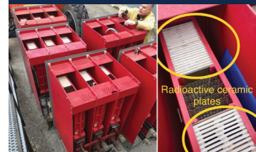
Ceramic Plates Inside Electrical Switches
