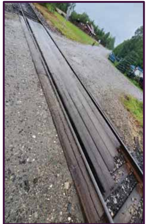
Figure 10: Crossing in Poor Condition
