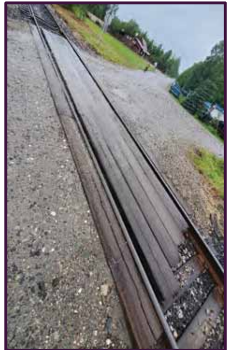
Figure 10: Crossing in Poor Condition
