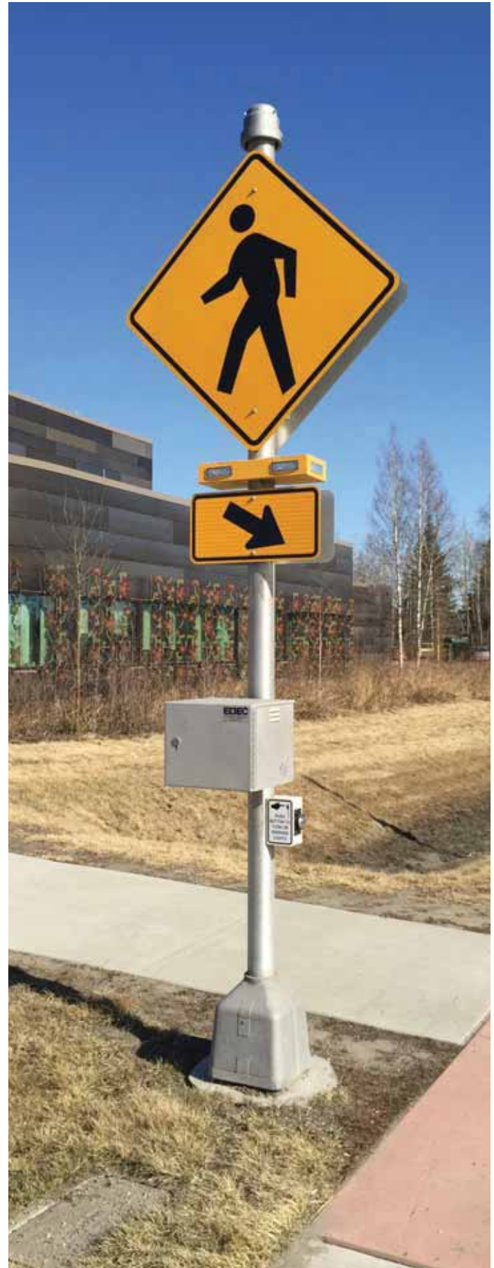
R&IP-Figure 1: Rectangular Rapid Flashing Beacon on Lathrop Street
