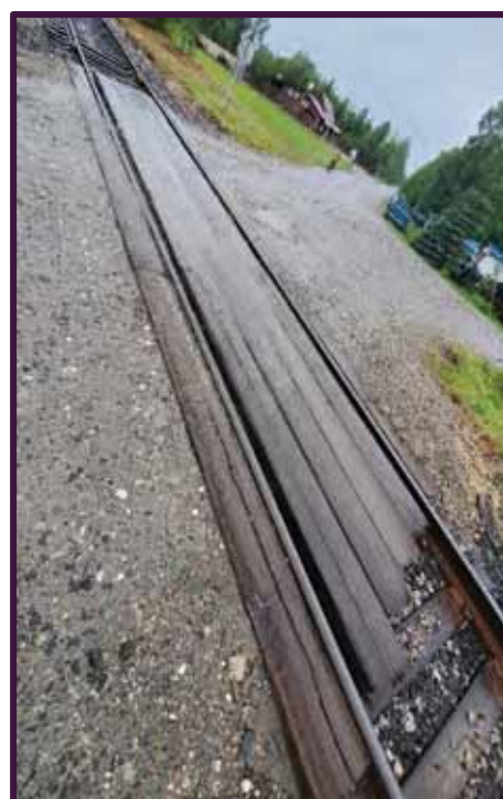
Figure 10: Crossing in Poor Condition
