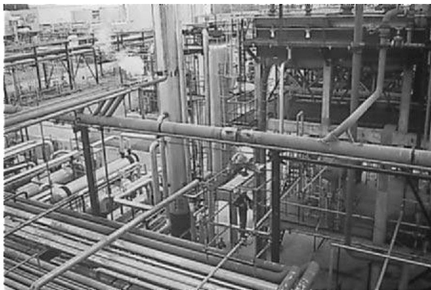
FIGURE C7.3 Typical process plant piping.
