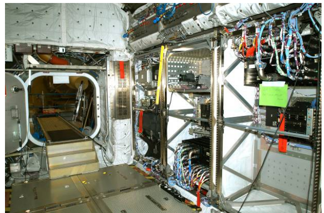
Columbus subsystem racks during testing
